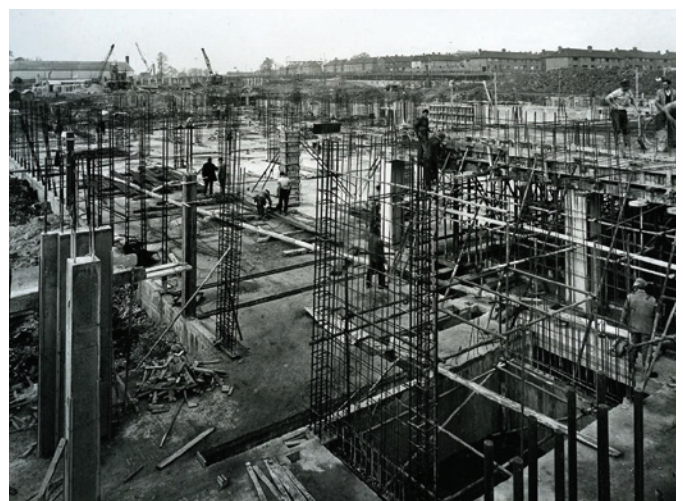
Figure 5 The new housing estate is visible in the distance, on the other side of the Central Line tracks. Building work in progress at the Debden Printing Works , May 1956 (Bank of England Archive, 15A/13/6/2).
